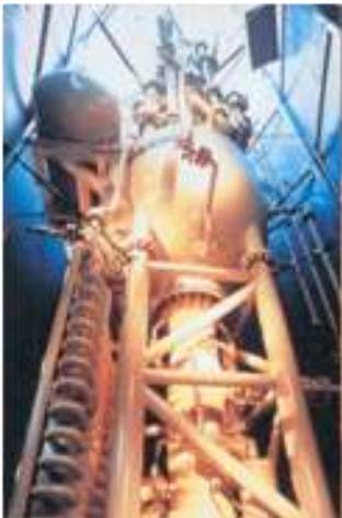
Booster station (KBS)
